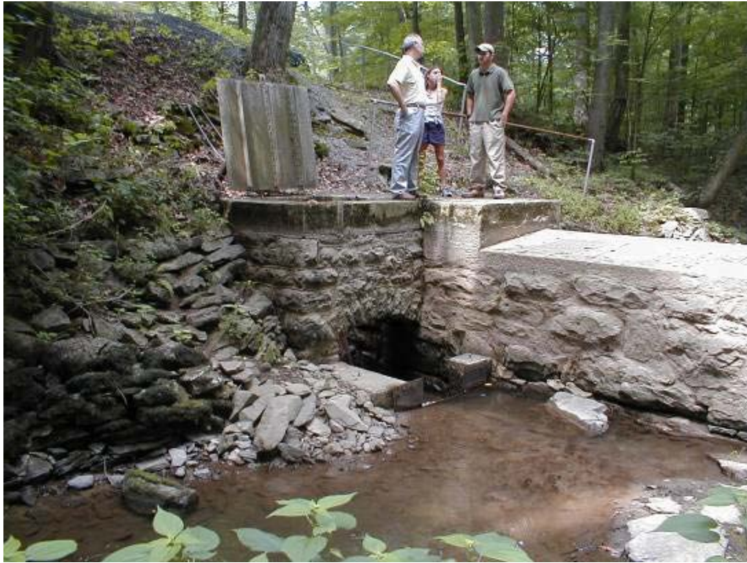
Hagerstown – Edgemont Reservoir, Raven Rock Diversion
